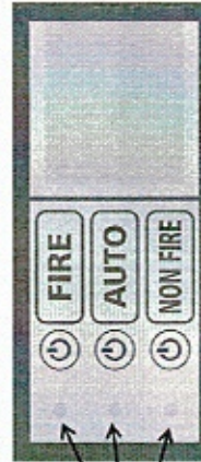
Damper Switch Position (Green LEDs)
